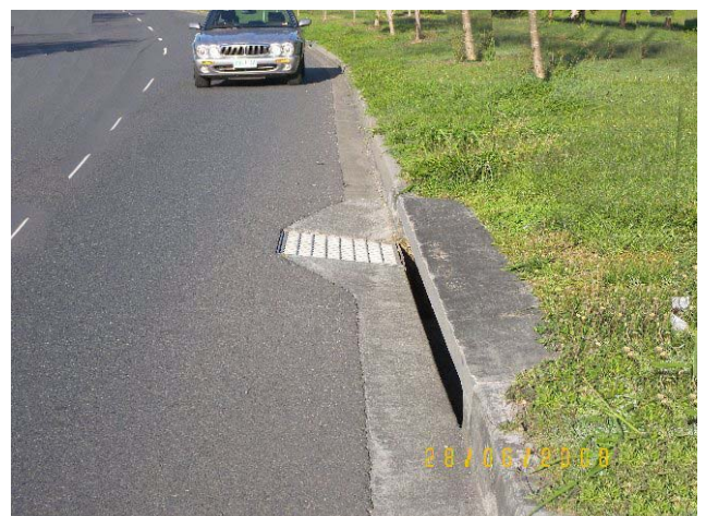
BCC inlet – large protrusion and depression
