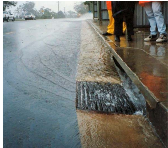
Manning grate capturing roadway flow
